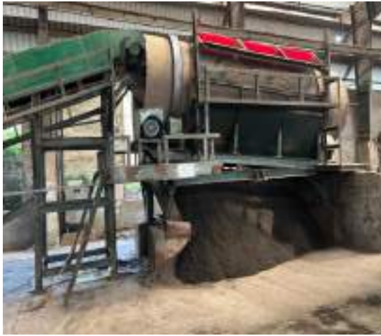
Figure 11 A: Composting trommel
