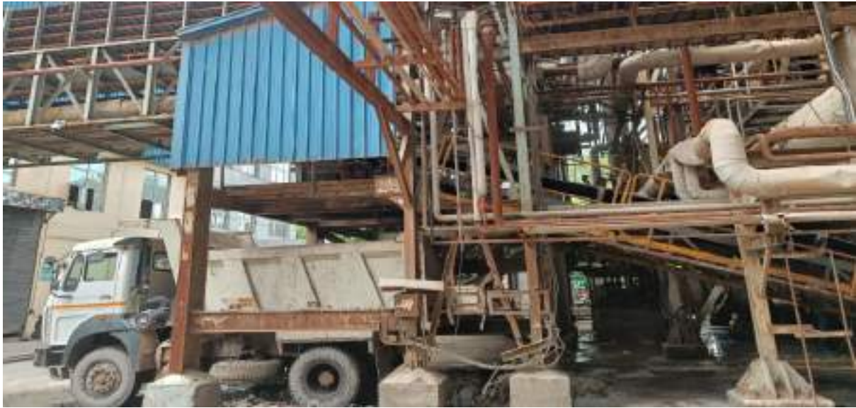
Fig 18: Bottom Ash handling
