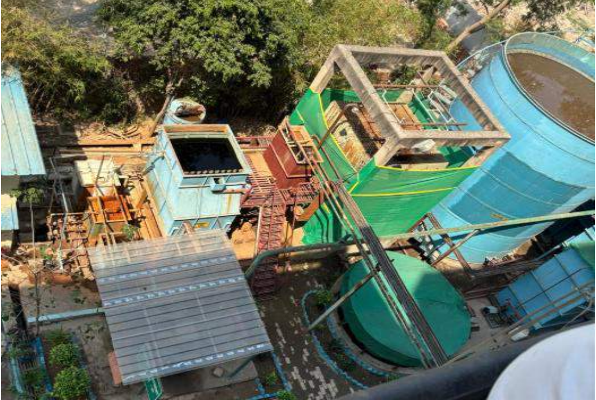
Figure 16: A Leachate Treatment Plant
